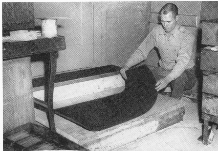
There's little danger of injuries due to falls on this stair platform where Robert Taylor (Carpenter Shop) is shown applying a non-skid grit surface. He's careful to get the grit surface flat so all the edges will be smooth.
